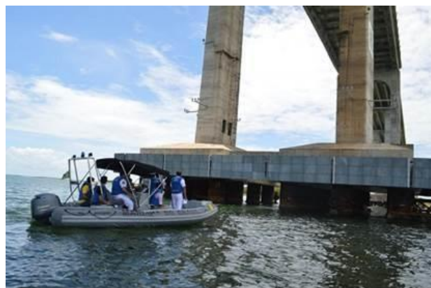
Figure 3 - Inspection on the pillars of the Newton Navarro bridge. Source: collection of authors (2017).
