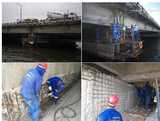
Figure 11 - Construction site for the refurbishment of the Igapó Bridge. Source: collection of authors (2019).
