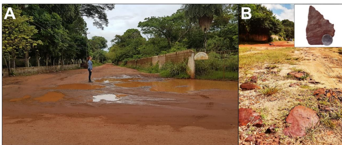
Figure 2 – (A): Location of permanent flooding on Rua Vera Paz in front of the access guardhouse to the UFCPA Campus Tapajós; (B): Outcrop of ferruginous concretion along the geophysical alignment with detail for Laterite sample.
