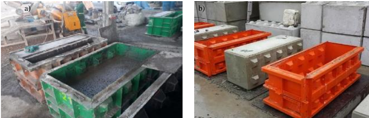
Figure 11 – Modeling and concreting of blocks a) concreting b) the concrete block Source: Authors (2019).
