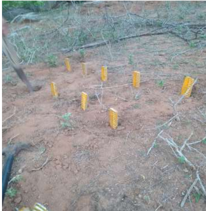
Figure 4 – Pins in the process of being installed at station 01. Source: Research data (2022).
