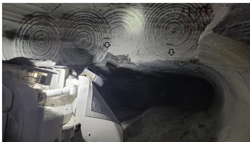
Figure 5 – Crack found in geotechnical survey. Source: Authors (2023).
