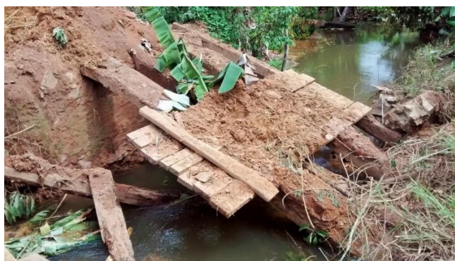
Figure 15 – Bridge destroyed by the waters of the creek. Source: Fieldwork (2015).
