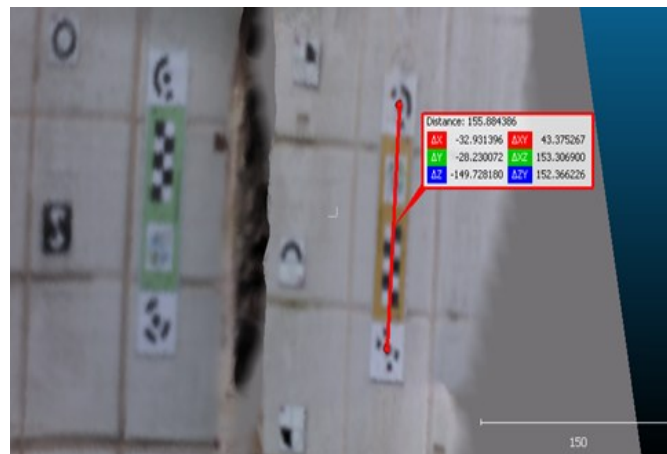
Figure 7 – Crack and measuring devices. Source: The authors (2026).
